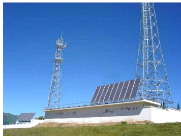
communication base station
