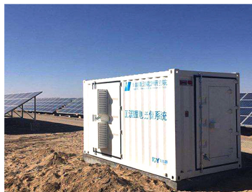
Energy storage system
