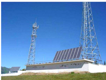
communication base station
