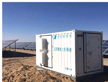
Photovoltaic energy storage system
