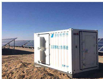
Photovoltaic energy storage system
