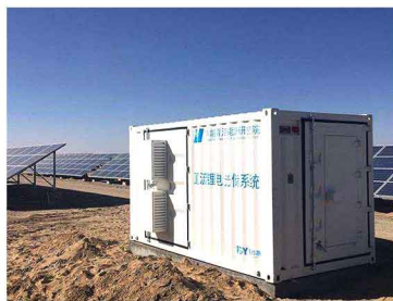
Photovoltaic energy storage system
