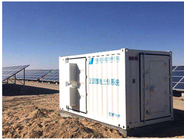
Photovoltaic energy storage system
