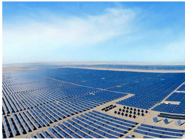
Photovoltaic power station
