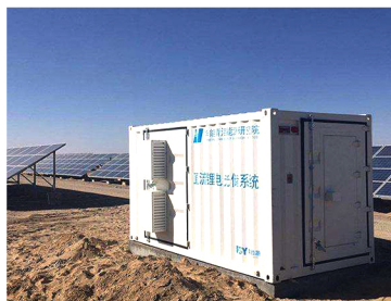
Photovoltaic energy storage system
