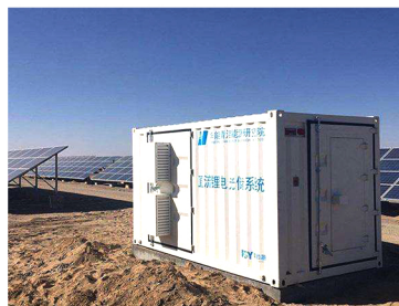
Photovoltaic energy storage system
