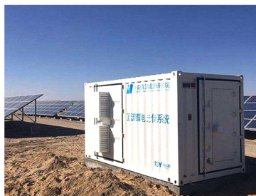
Photovoltaic energy storage system
