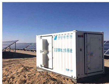
Photovoltaic energy storage system
