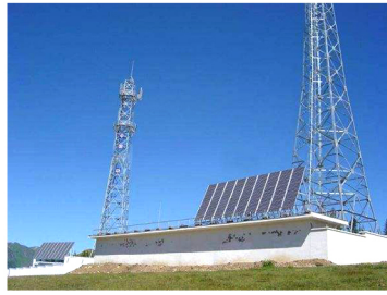
communication base station
